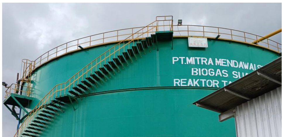
Figure 36. SSMS's 1.5 MW biogas plant
