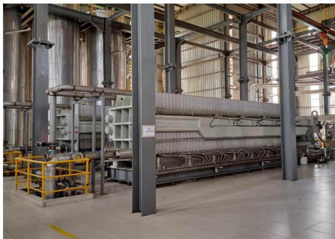
Figure 26. STAOF fractination installation
