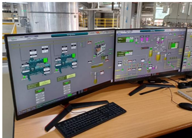
Figure 27. STAOF control room monitoring system
