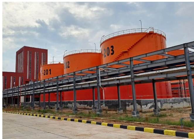
Figure 29. STAOF storage tank
